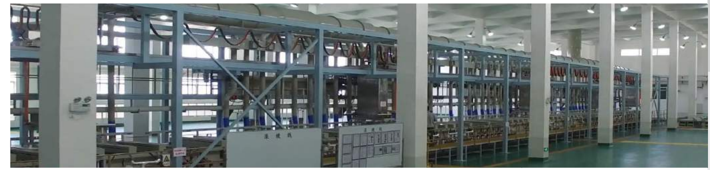
Surface Treatment Line
